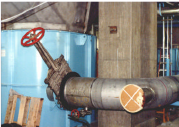
Trim Effluent Line Entering Pulper
