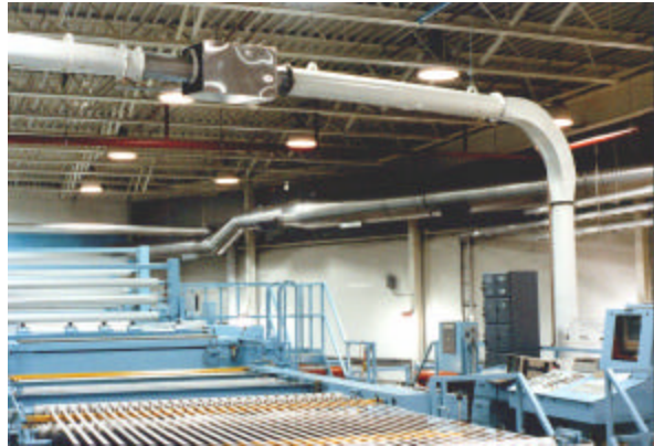
Ductwork with Airflow Control Valve over Folio Sheeter
