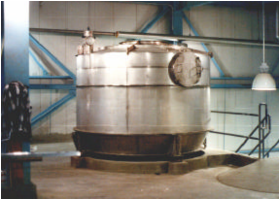
Trim Separator on Mezzanine
