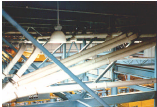
Ductwork in Trusses
